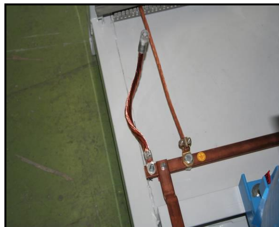
Fig. 13.- Ground connection between modules
