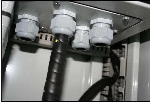
Fig. 16.- Stuffing boxes for control cables
